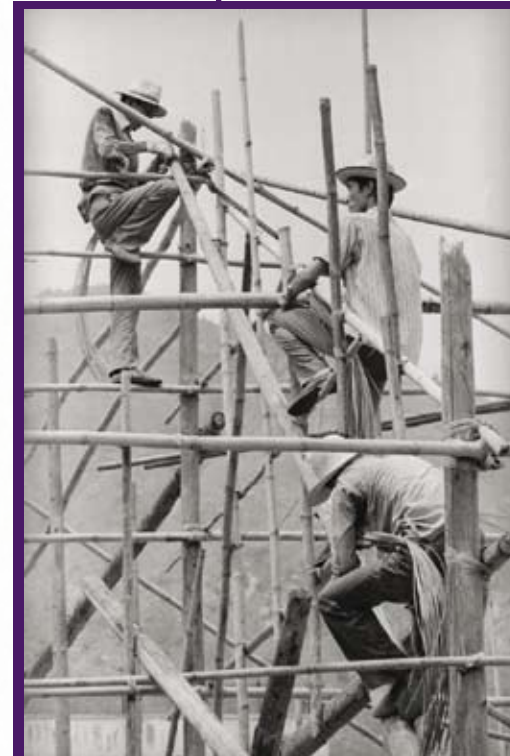
傳統的搭棚技術一直是建造工程的重要環節 Traditional scaffolding has always been an important part of construction works
