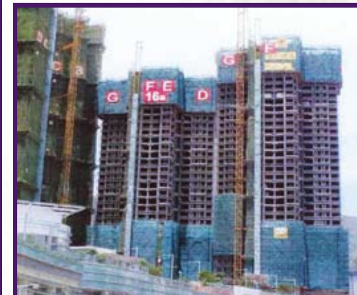
今天爬升棚架已被普遍使用，顯示傳統技術不斷改進。 Climbing scaffoldings that are now widely used demonstrate continuous improvement of traditional technology
