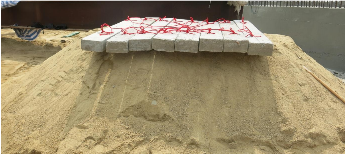
Photo E3 Concrete strips placed on backfilled sand above J1 well to strengthen the protection
