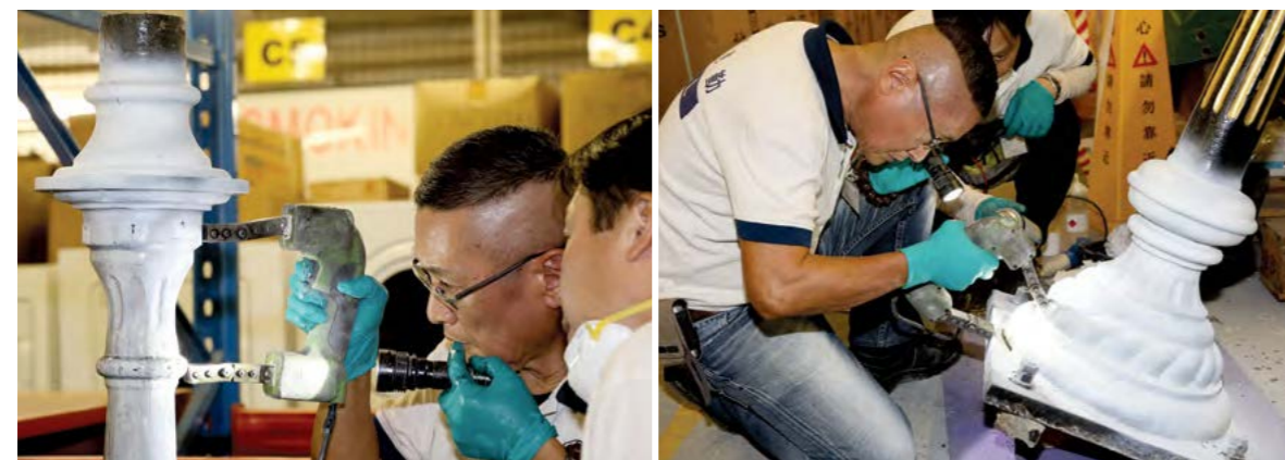
Fig. 21 A specialist contractor conducts a non-destructive test on the two cast-iron columns at the Towngas store.
