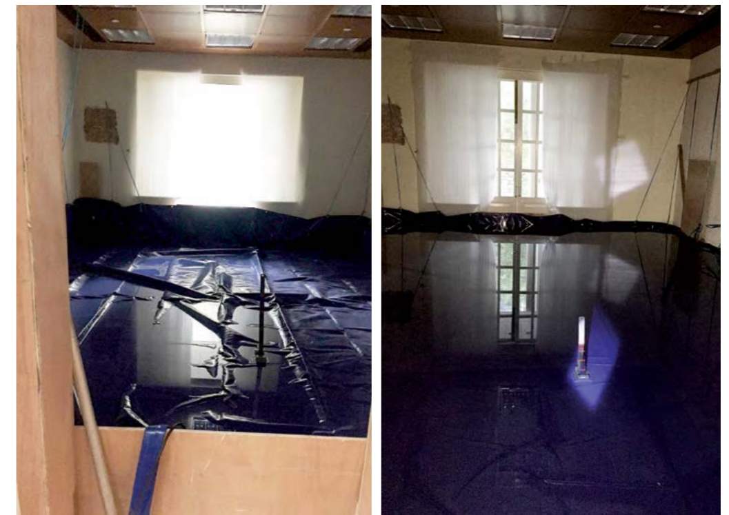
Figure 17 Loading test carried out in the room on the 1/F where the existing slab would be demolished for the construction of the new escape staircase. [Source: Hop Lee Builders Company Limited]
