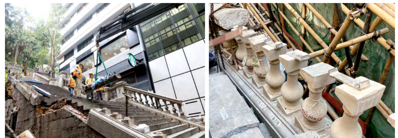
Fig. 19 With reference to the reinforcement method previously adopted on-site, U-shaped stainless-steel plates were installed on the newly cast cement balusters to reconnect and reinforce the broken granite handrails.
