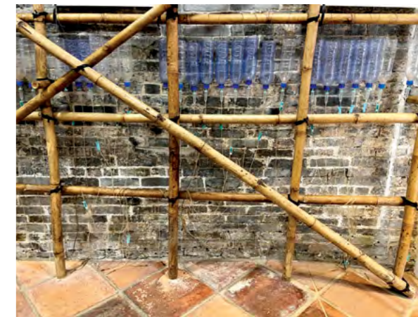
Figure 13 The Damp Proof Course Injection - Former Chong Sai Pharmacy Source: Photo taken by Kong Ka lan
