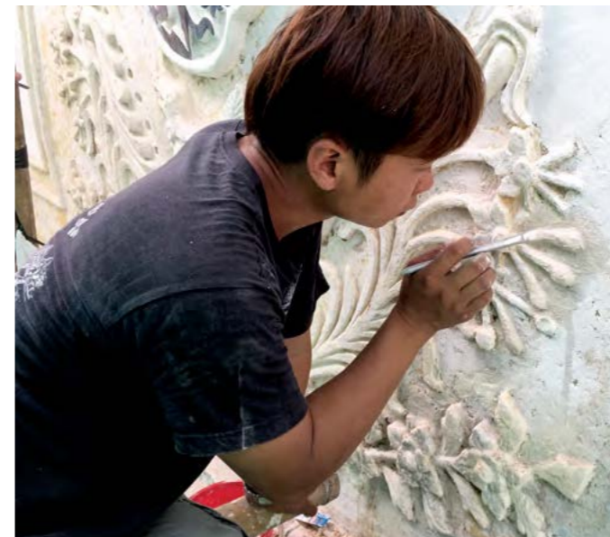
Figure 9a Heritage Guard Program - Lime stucco restoration in the St. Dominique Church Photo taken by author
