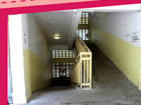
H型和I型的工廠大廈高六至七層，沒有升降機，要利用建築物中間的斜道搬運貨物。 H-shaped or I-shaped factory estate, 6 or 7 storey without lift machine, the ramp on the middle was used for moving goods
