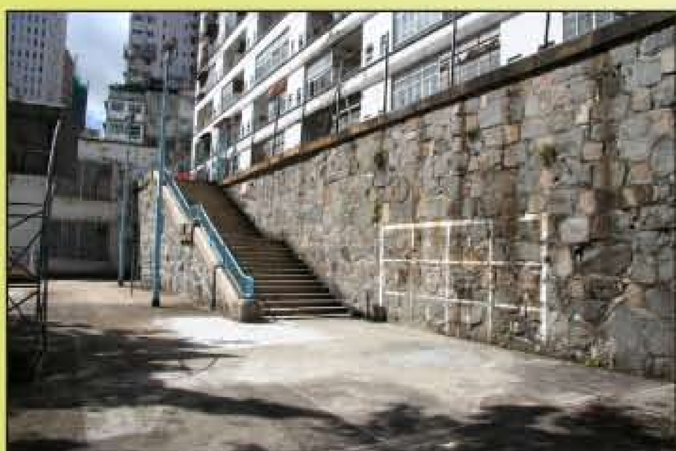
連接第二及第四平台的一段花崗岩石級和粗石擋土牆 A flight of granite steps linking the second and fourth plateaus, and the rubble retaining wall
