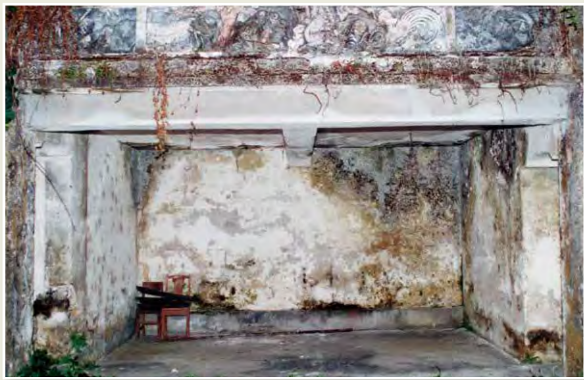
修復前的前院廂房及女兒牆 The side chamber and parapet of the front courtyard before restoration
