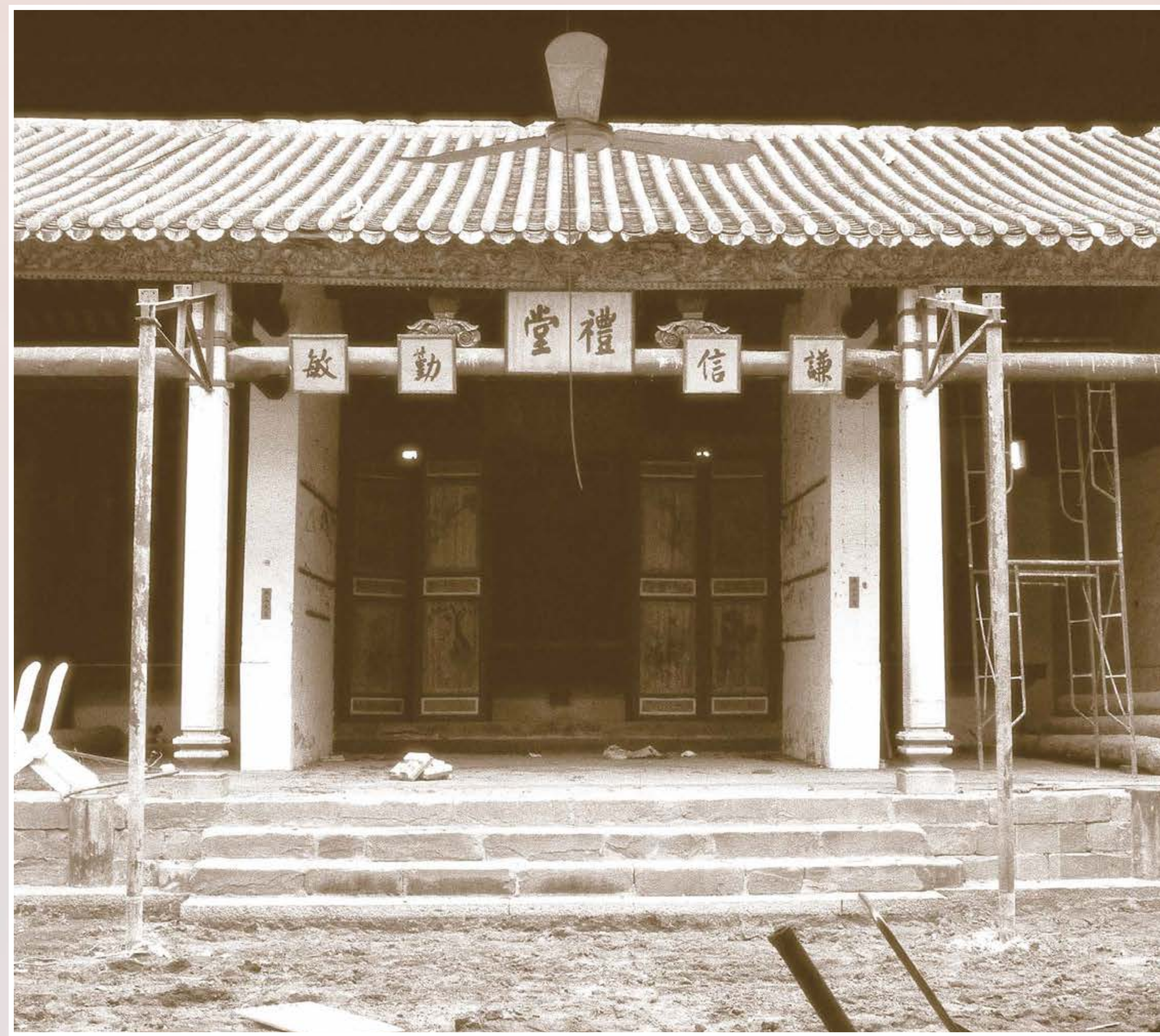
修復前的廖萬石堂後進 The rear hall of the Liu Man Shek Tong Ancestral Hall before restoration
