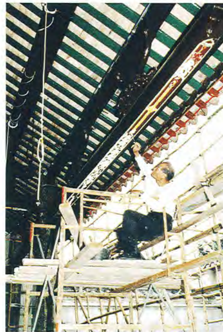
清樂鄧公祠正進行大規模修葺 Major repair work is being carried out to Tang Ching Lok Ancestral Hall.
