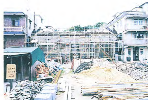
敬羅家塾維修工程即將展開 Restoration of King Law Ka Shuk Ancestral Hall about to commence.
