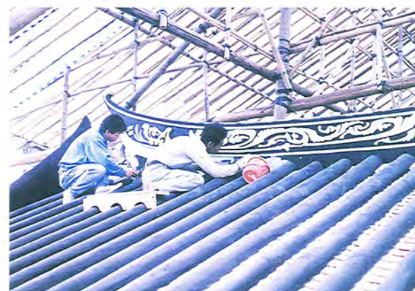
張氏宗祠修繕工程 Restoration work in progress at the Cheung's Ancestral Hall.
