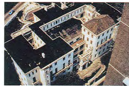
46. 半山區列提頓道聖士提反女子中學主樓 Main Building of St. Stephen's Girls' College, Lyttelton Road, Mid-Levels
