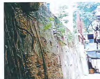
至今仍保留的一八九五年諾士佛臺下的護土牆 The surviving part of the 1895 retaining wall below Knutsford Terrace
