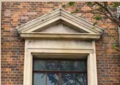
鐘樓上的長方形玻璃窗，配以木框、花崗岩窗框和三角形楣飾 The rectangular glass window on the Clock Tower has wooden-frame, granite window surrounds and pediment window head
