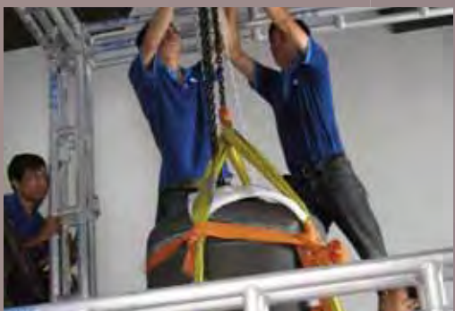
2010年大銅鐘安裝於鐘樓內 Installation of the Bell at the Clock Tower in 2010
