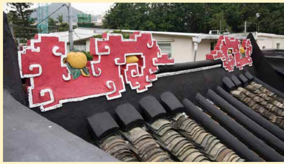
屋脊兩端的夔龍灰塑 The plastered reliefs of kuilong at the ends of the ridge
