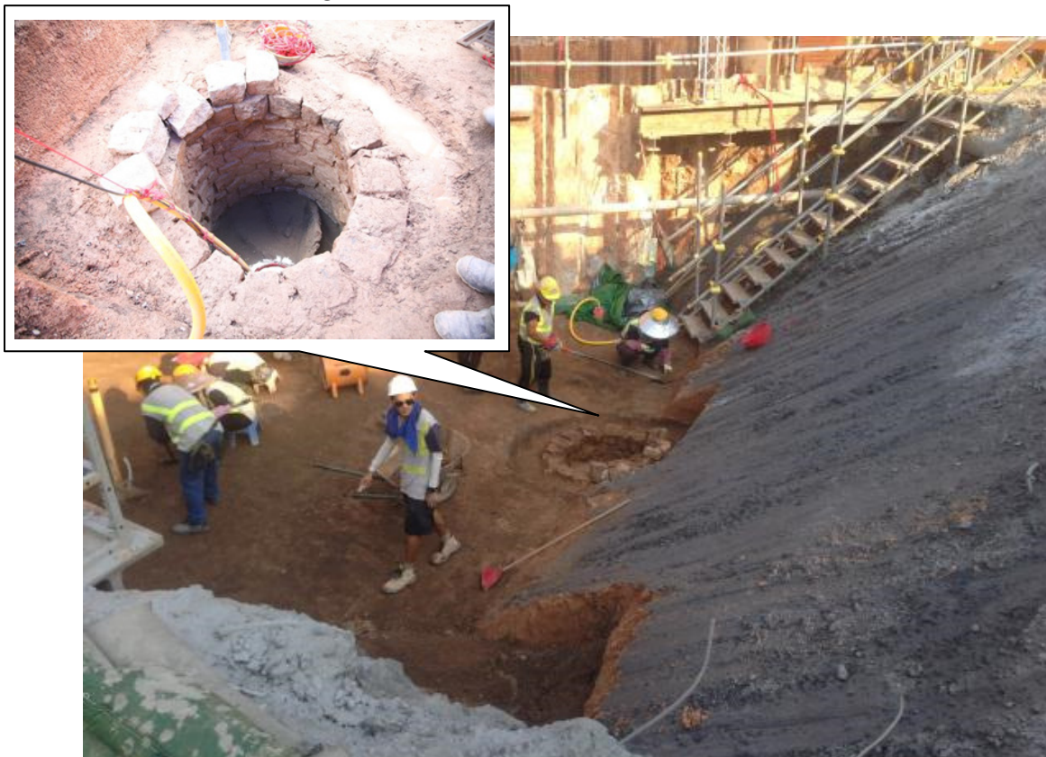
Photo 4: A well of Qing to Republican periods was discovered in the area between Ventilation Shaft and Adit C (Zone D).
