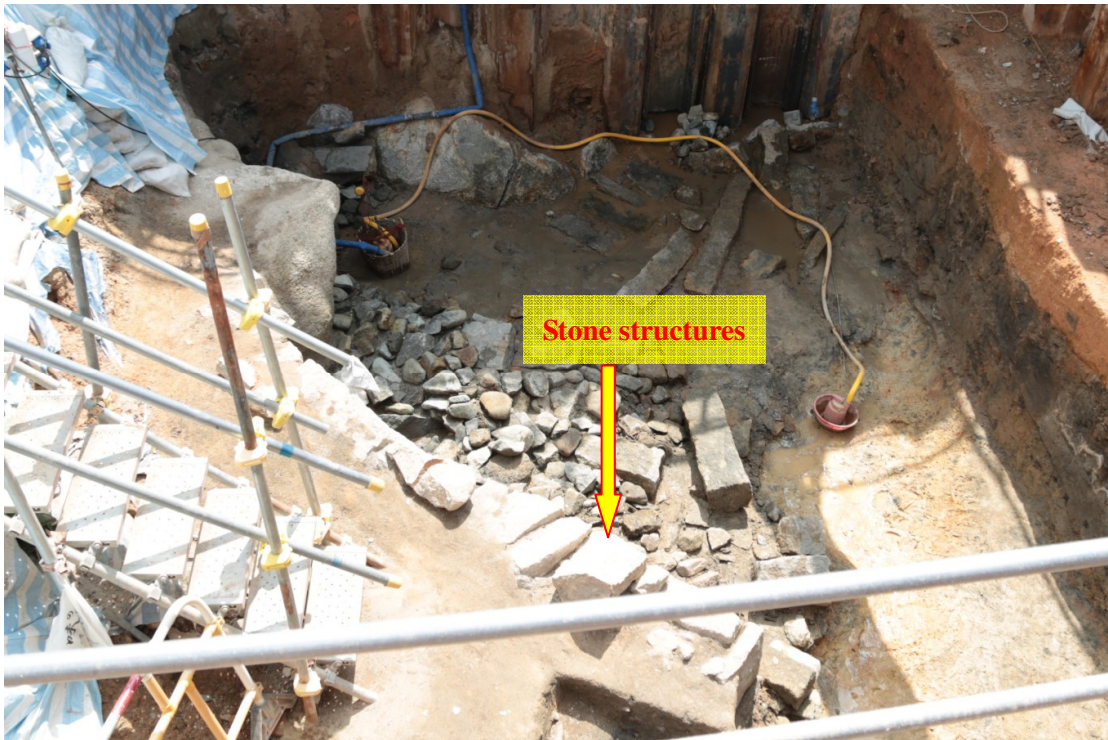
Photo 3: Stone structures of the late Qing to Republican period which formed the riverbank of the former Ma Tau Chung were revealed.
