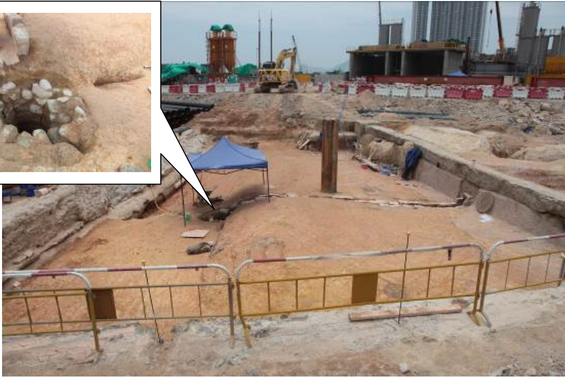
Photo 6: Archaeological remains of a water channel system was discovered below the fill layer
